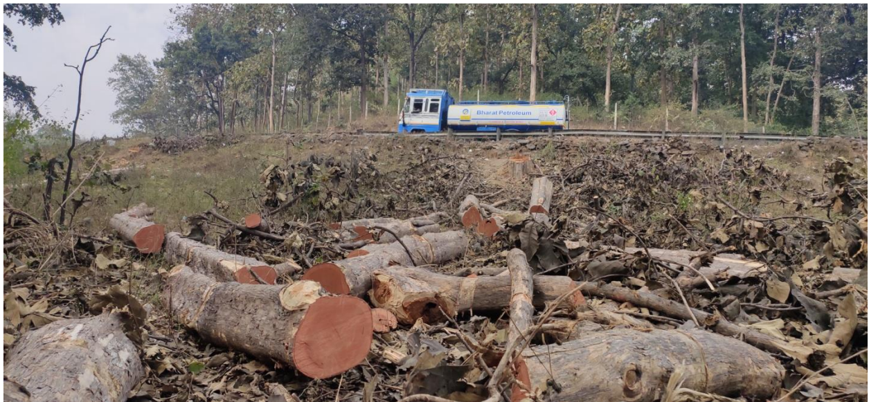
Photo: Road Expansion Causing Tree Cutting in Forest Area.
